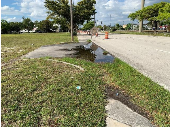
The vacant parcel/former development on the west side of Dixie Highway between SW 4 th Street and SW 3 rd Street driveway is unmaintained, which causes discontinuation in the sidewalk with overgrown grass and flooding.
