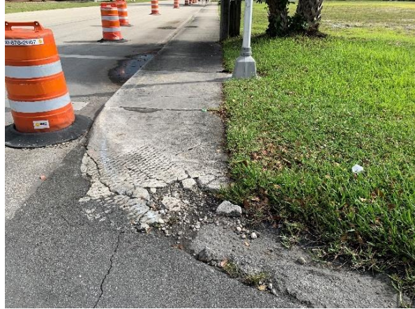
Sidewalk cracking which causes trip hazards.
