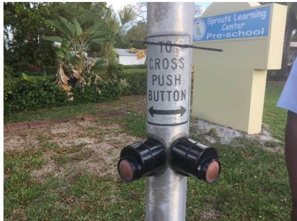
Outdated pedestrian pushbutton at Sprouts Learning Center Pre-School located at the southeast corner of SE 1 st Avenue and SE 3 rd Street.
