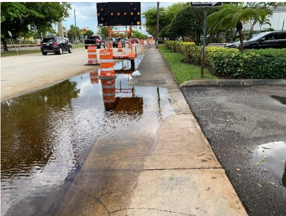
Drainage issues along Dixie Highway and SE 1 st Avenue, which causes excessive water over sidewalks.
