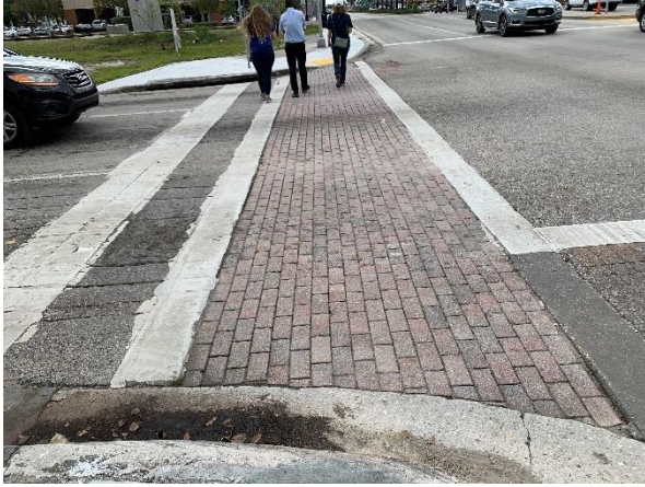
Concrete pavers used for crosswalks may cause rigid body uplift or settlement.
