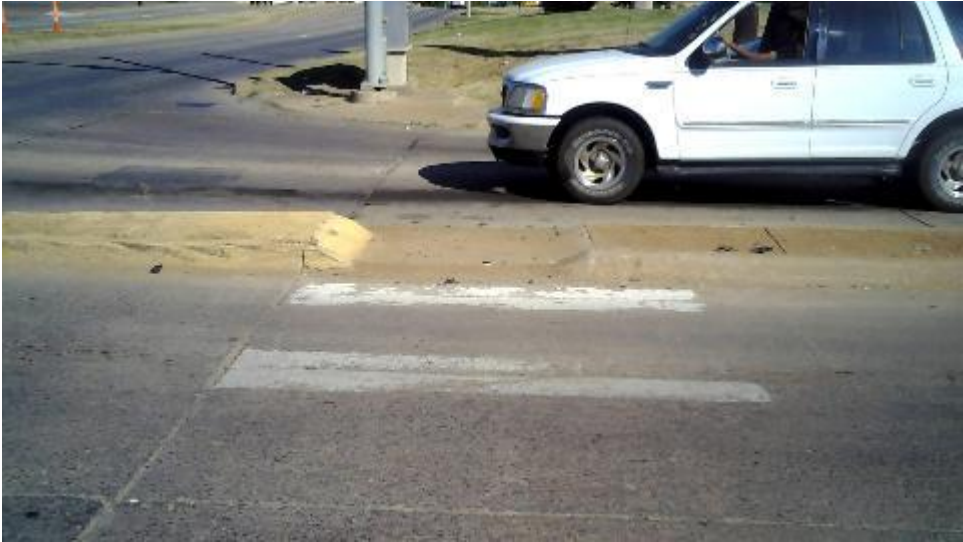
Non-compliant: Sides not 90°
