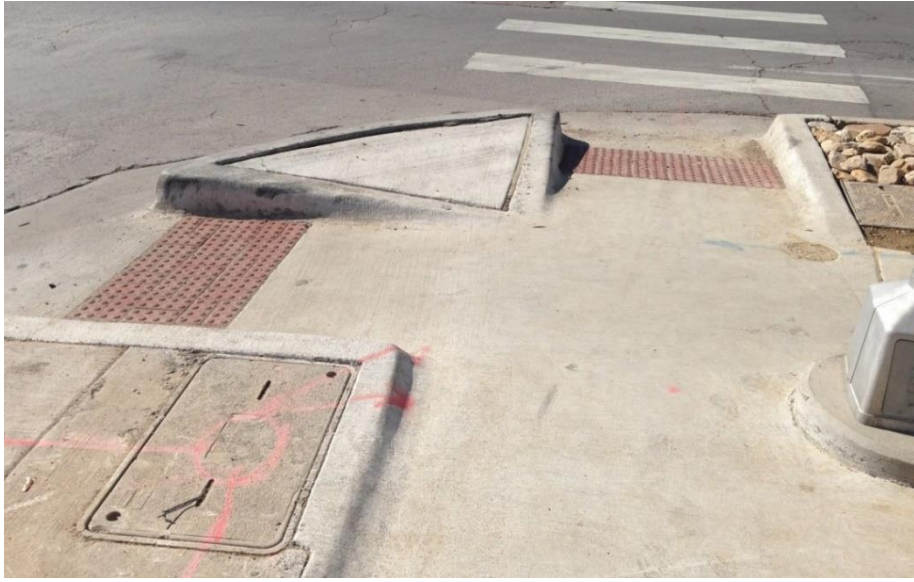
NON-COMPLIANT (traversable adjacent surface)
