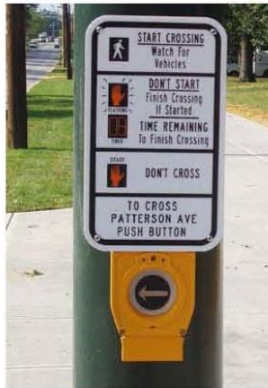
Pedestrian Activated Signals
