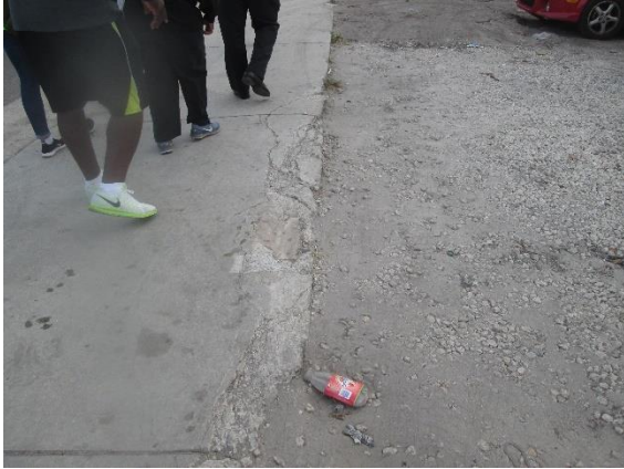
Cracked sidewalk/trip hazards along the sidewalk.
