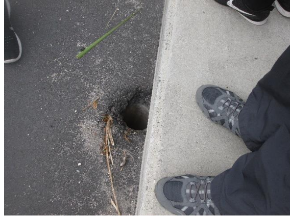
The open pipe is exposed for potential sediment build-up.
