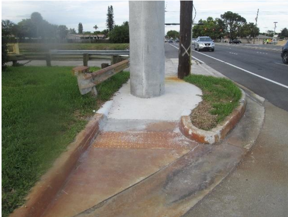
Street fixtures are within the sidewalk near the driveway entrance to International Cold Storage which is hazardous for non-motorized users.
