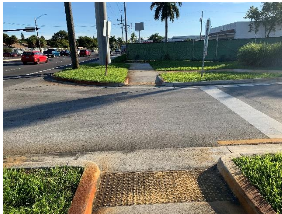
The driveways along the corridor are unmarked crosswalks.
