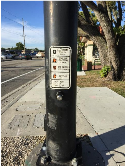
The MUTCD R10-33 (Traffic Signal Pedestrian) sign is shown to be slightly damaged at the northeast corner of NW 31 st Avenue and NW 39 th Street.
