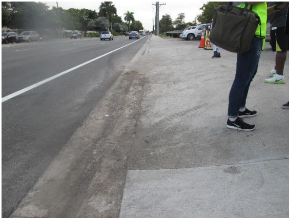
The driveways may cause hazardous drop-offs and needs to be upgraded to standard.
