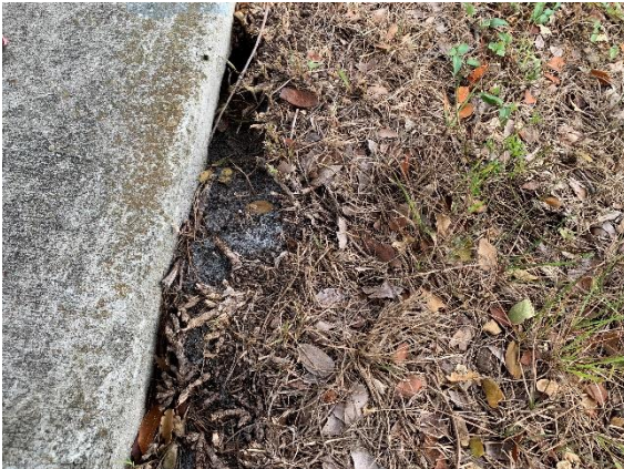
Soil wash out/erosion of subbase underneath concrete sidewalk.
