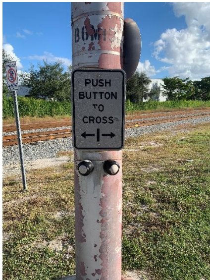
SR 811/Dixie Highway and SW 4 th Street pedestrian push buttons in the southeast corner did not function.
