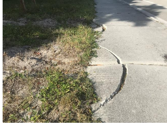
Concrete sidewalk cracking which causes trip hazards.
