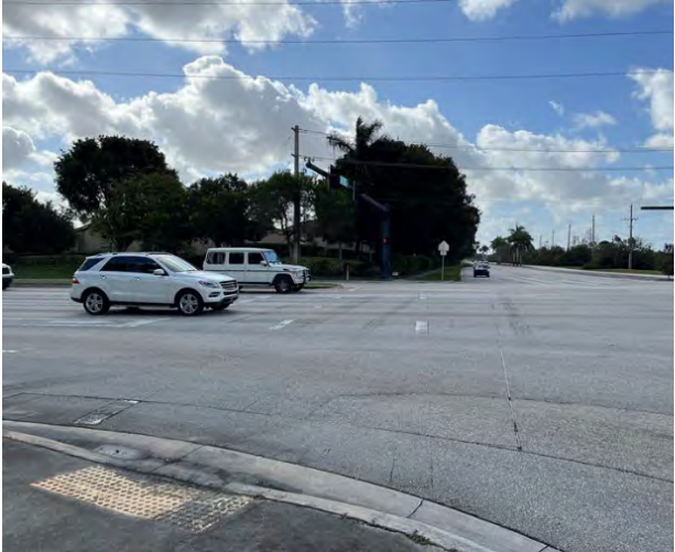
Crosswalk at SW 172 nd Avenue needs re-striping and audible signals.
