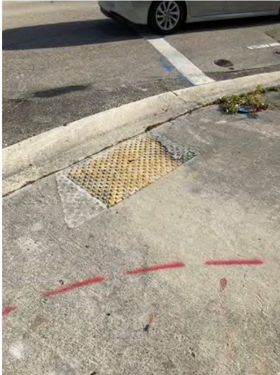
Outdated and worn ADA detectable warning surface at the SW 160 th Avenue intersection.
