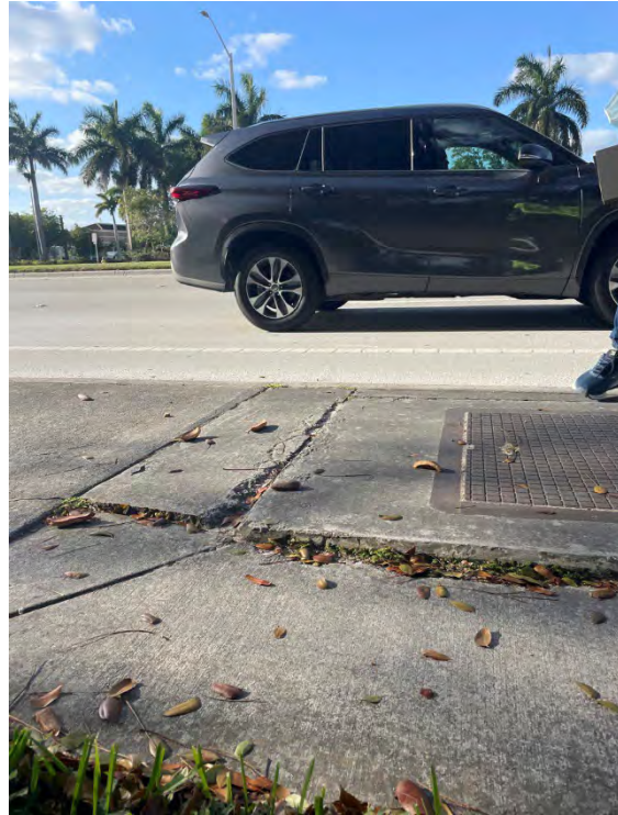
Observation 28: “Raised utility cover where concrete has settled unevenly around the covering.”
