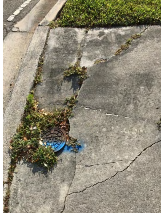
Cracked and vertically deflected sidewalk at the SW 160 th Avenue intersection.
