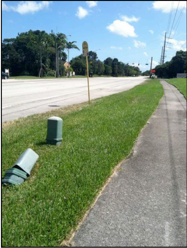
Photo 23: Examples of Broken Electrical Boxes and Bus Stop Without Amenities or ADA Facilities
