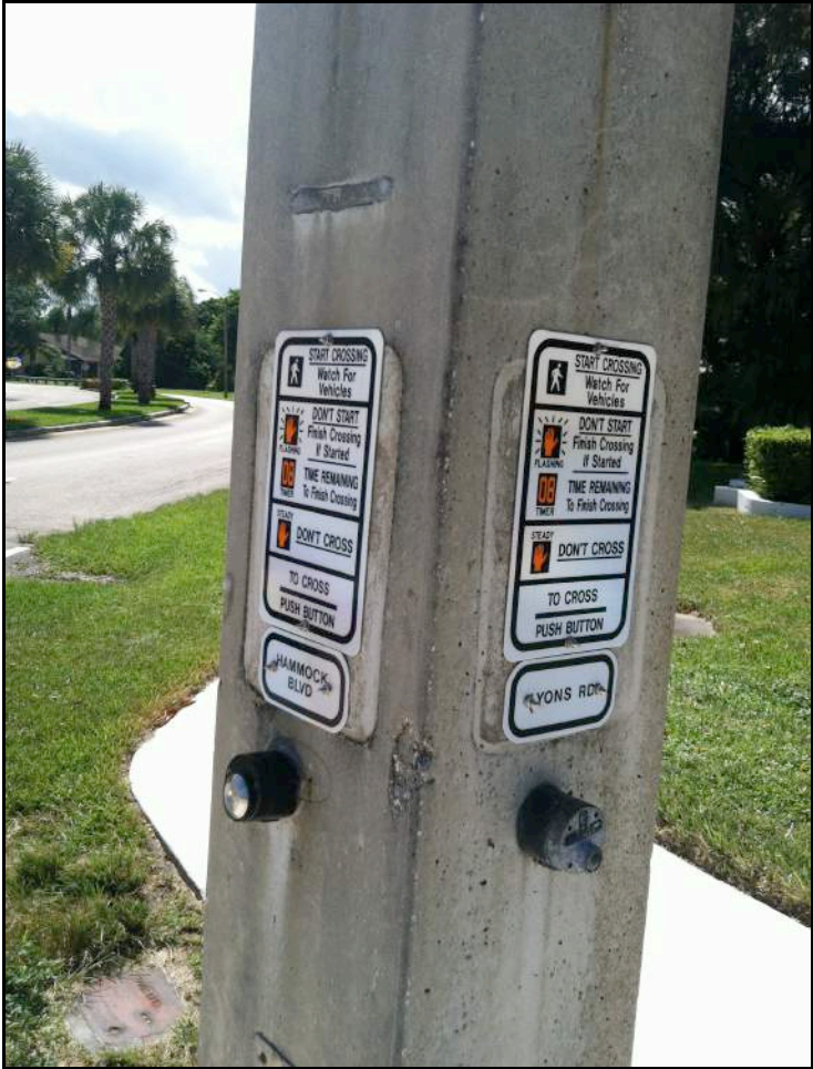
Photo 19: Pedestrian Push Buttons and Signage at Lyons Road and Hammock Boulevard
