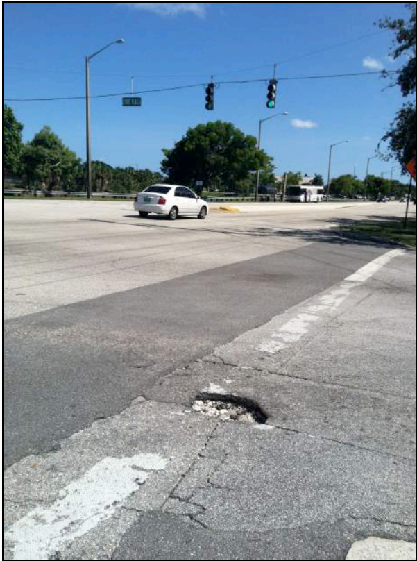
Photo 11: Pothole on the NW Corner of Lyons Road and Lyons Plaza
