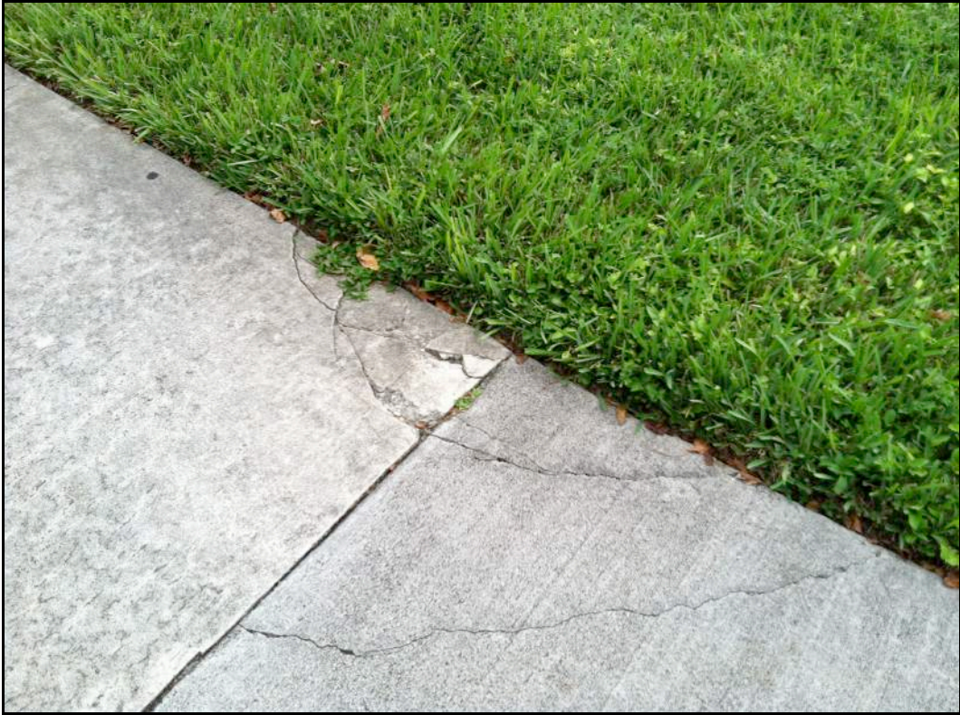
Photo 09: Example of Cracks in the Sidewalk, Along Lyons Road
