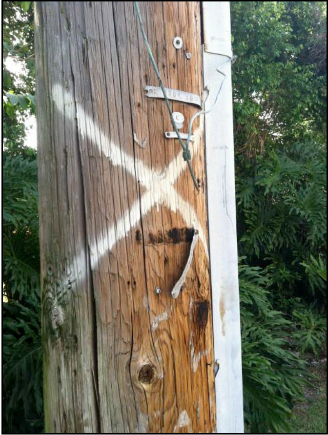
Photo 15: Wooden Utility Pole with Loose Metal Pieces, West Side of Lyons Road
